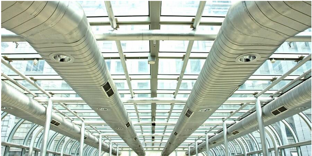
Fig- Oval Duct
